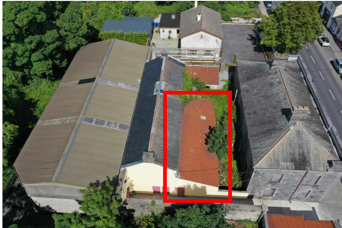
Demolition of Lean-to Extension on Adjacent Bridewell Unearthed Original Entrance Door & Windows
