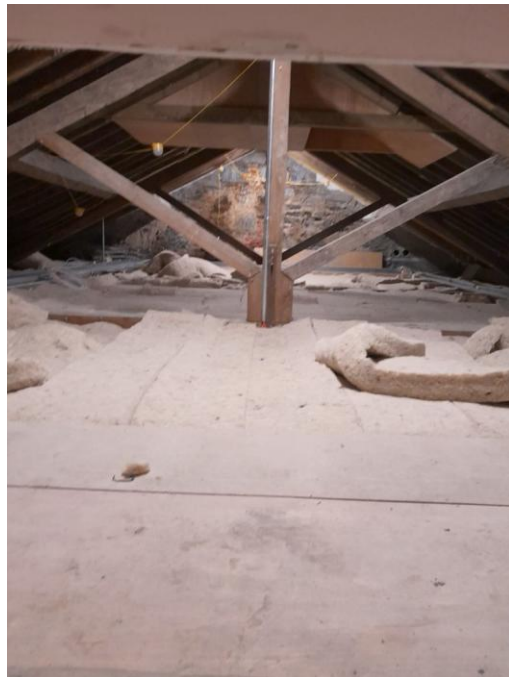
Sheeps Wool Attic Insulation
