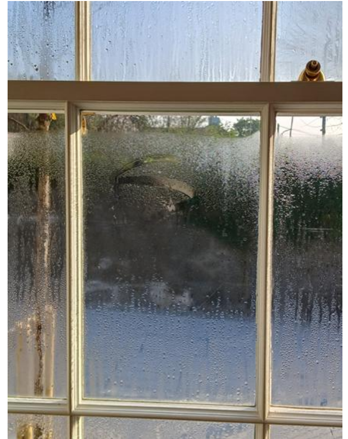
Condensation present on single glazed windows
